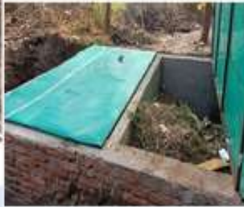
DRY AND WET WASTE MANAGEMENT
